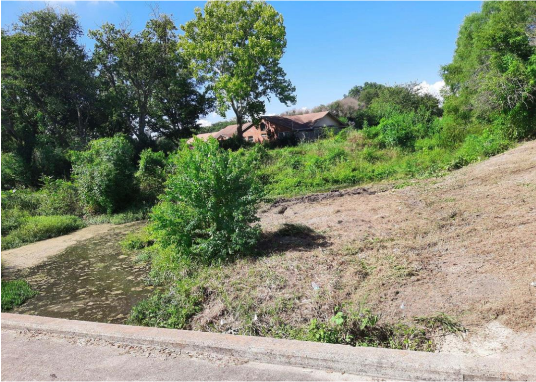
Before/After removing silt bottle neck at Castleman Creek Approximately 15- 8 yard truck loads of soil removed
