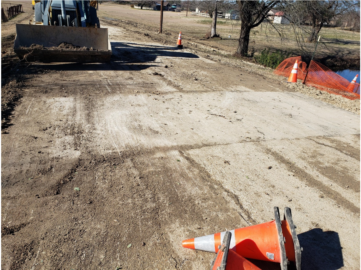
Base/Asphalt patched (dirty from shoulder dirt work going on at time of photo)
